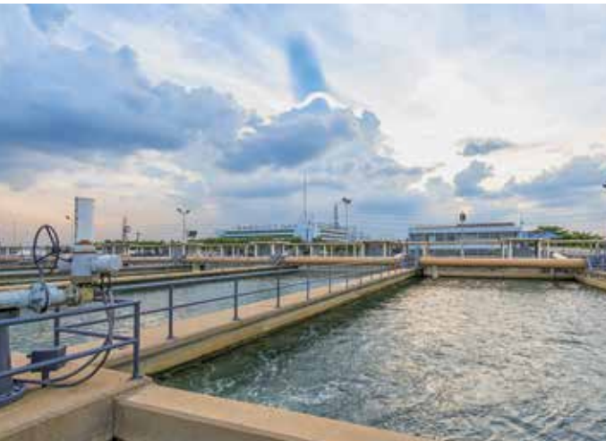
Waste Treatment Plants - Station d'épuration
